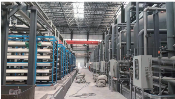
Wastewater reuse in coal chemical plant
